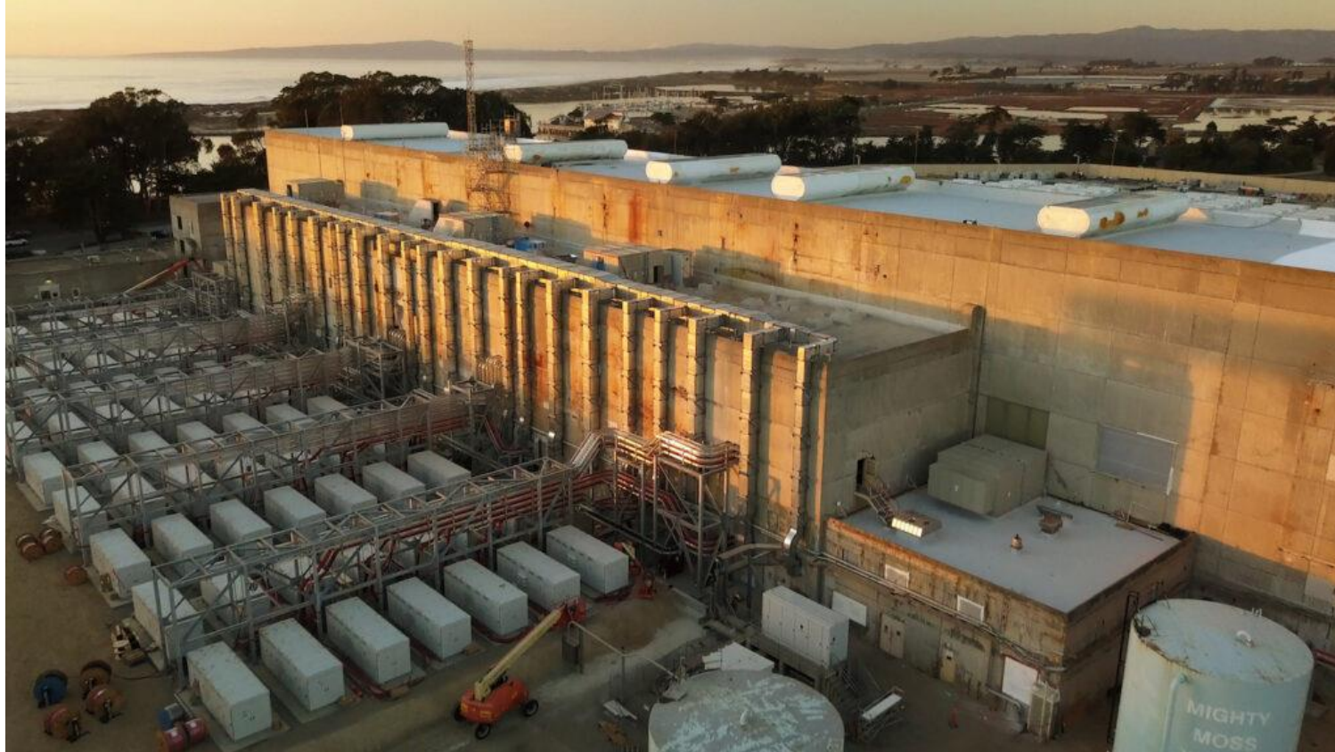
Vistra's 750MW/3,000MWh in California.
